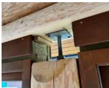
Figure 1. Difficult window detail (not sealed)
